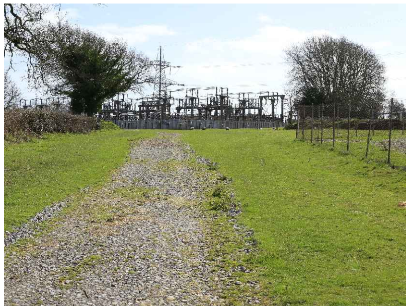
Axminster, Devon 400kv substation
