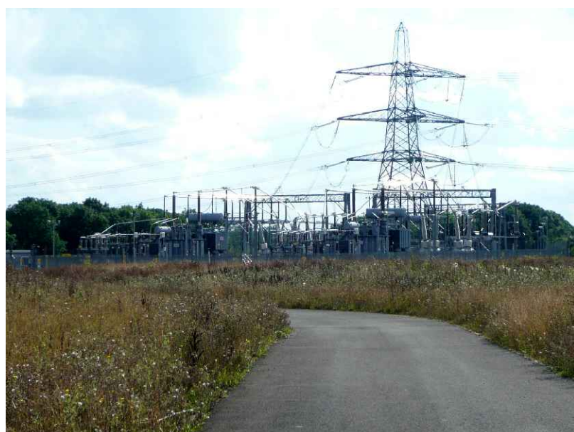
Ryhall, Rutland 400kv Substation
