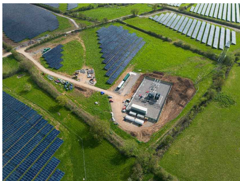
New Project Substation, Larks Green COPYRIGHT : ENSO ALEXPARKYNSMITH
